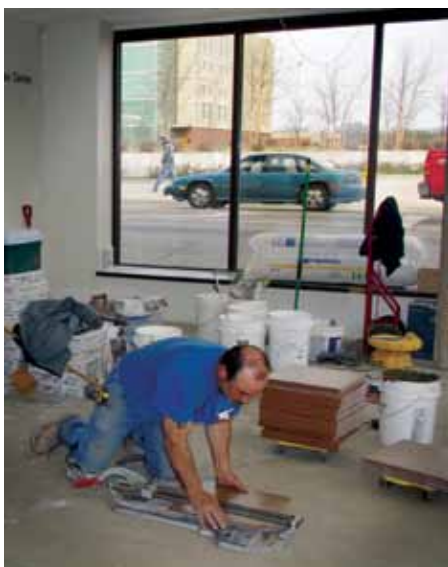
Workers install floor tiles in the entrance lobby at Janet Wattles Center on April 15.
